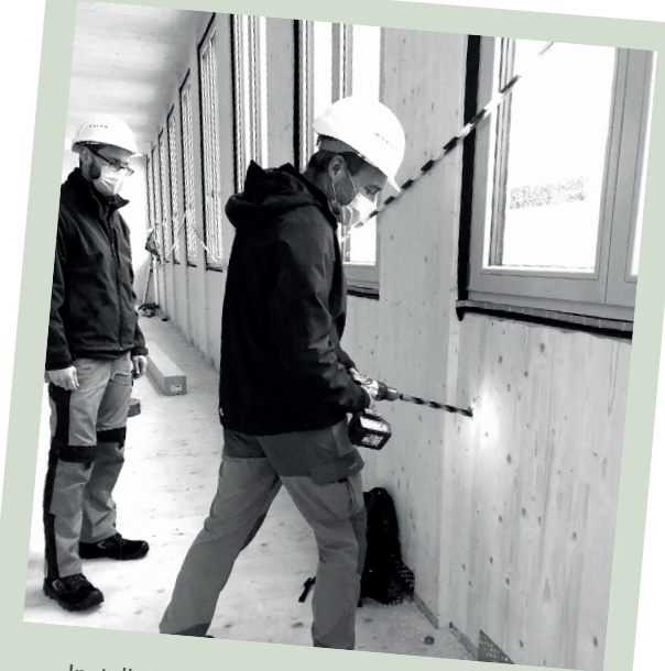
Installation of sensors for monitoring humidity in wooden walls and façades Montaža senzorjev za monitoring vlage lesenih sten in fasade
